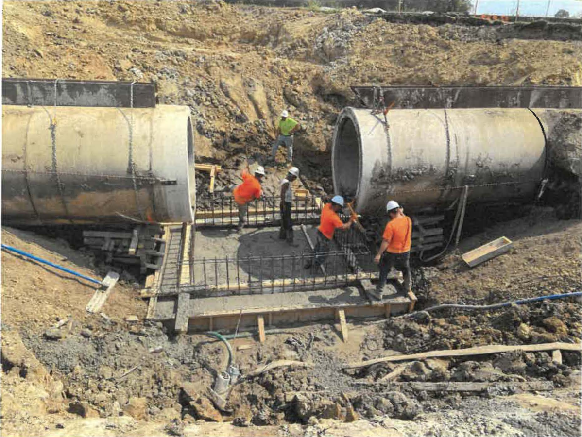
Sherman Sewer Diversion Structure
