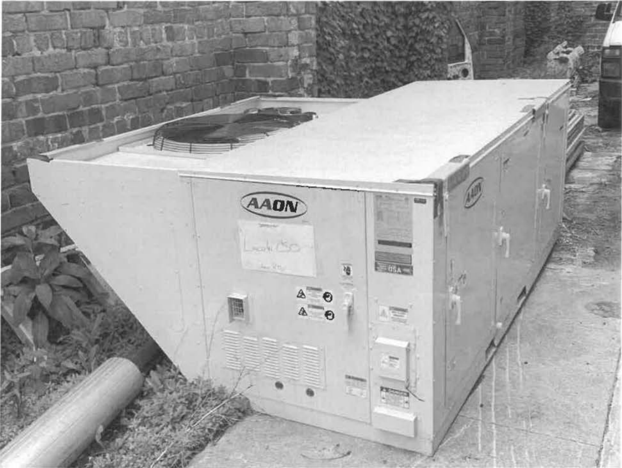
Lab Building RTU
