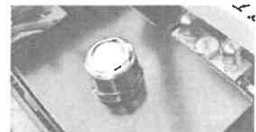
Large Oil Reservoir
